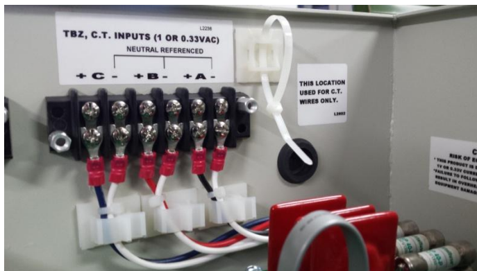
TBZ, Current Transducer Wiring Location
